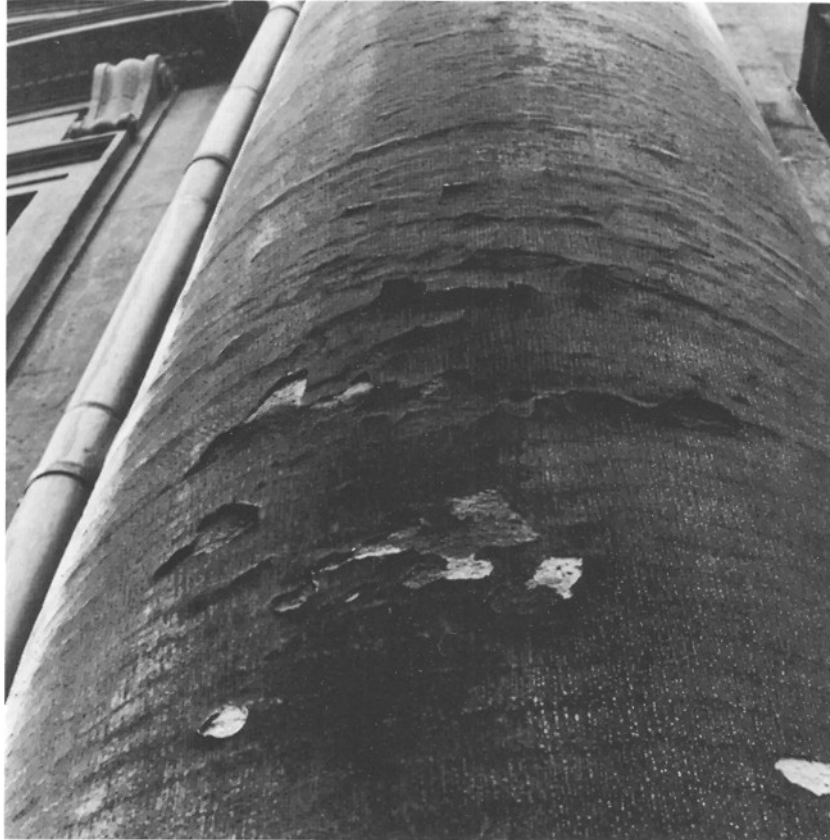
Fig. 1. The crackling and exfoliation of the black crust on one of the columns of the Marble Church in Copenhagen.
