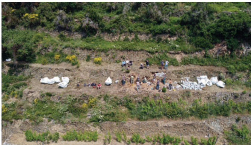
Dry-stone wall reconstruction and restoration in the Cinque Terre National Park © Parco Nazionale delle Cinque Terre (Emanuele Raso)
